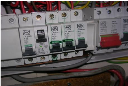
Goo leaking from a Consumer Unit.
