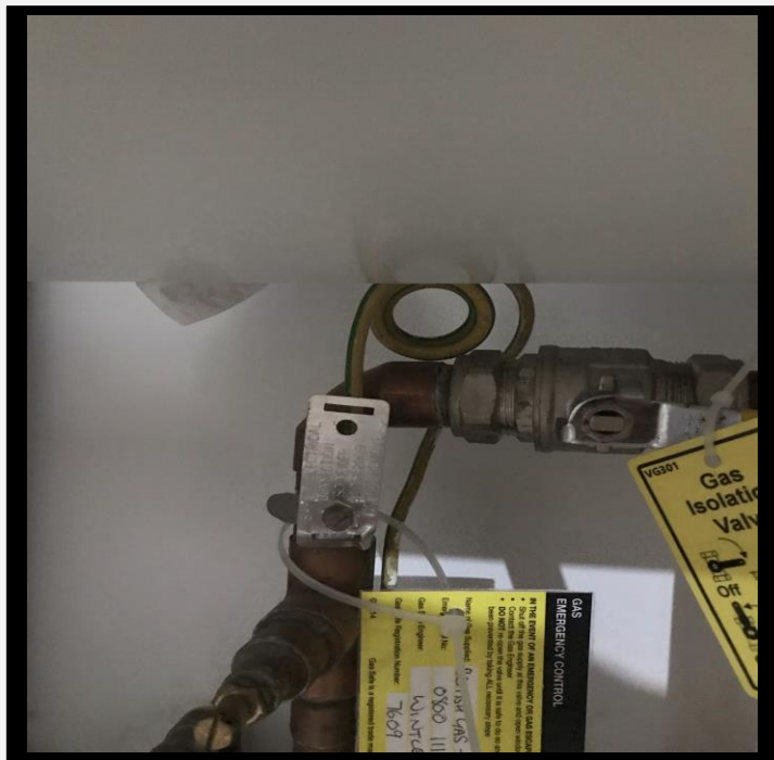
A typical Earth Bond and Clamp located at a Gas Meter
